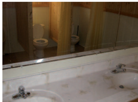
The first waterless urinal was installed in Rangers Cabin's new bathroom.
