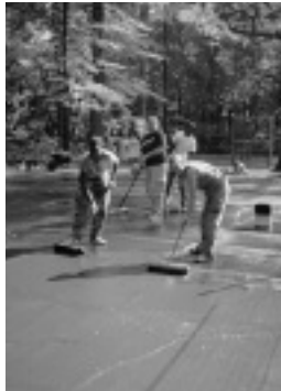
The hard surface volleyball & basketball courts get a new surface and upgraded fence.
